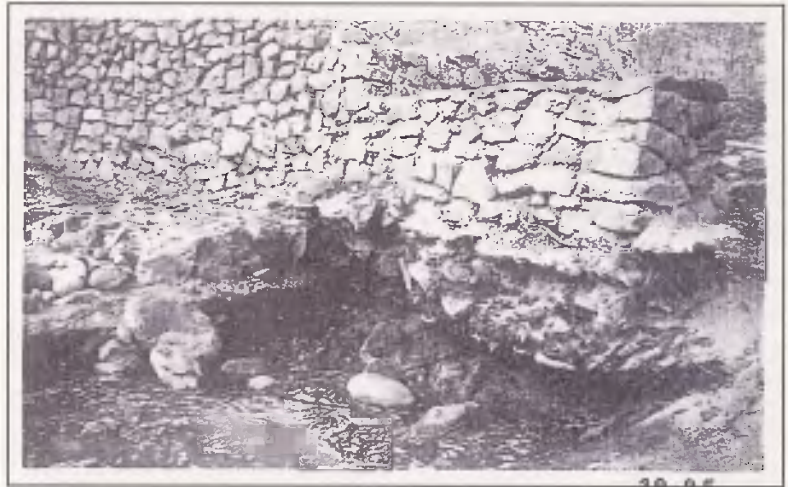
Damages from March 1938 flood showing eastern wingwall.
