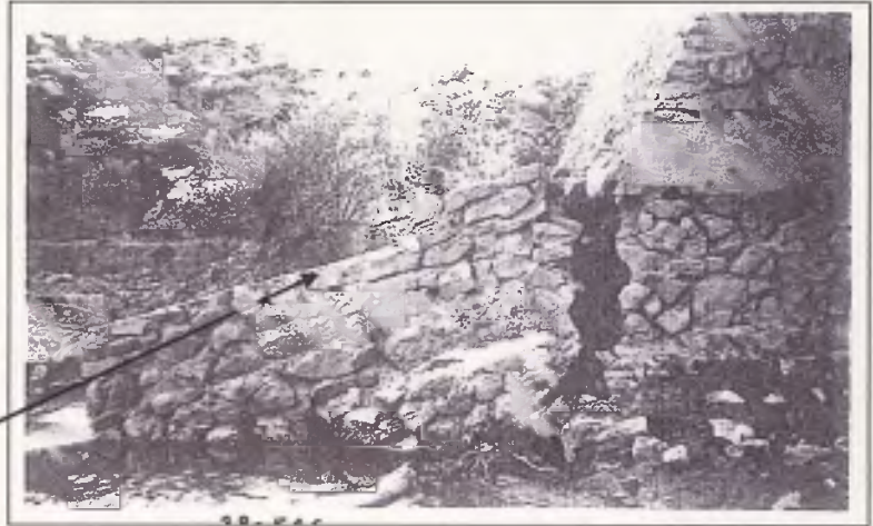
Damages from March 1938 flood showing western wingwall. The names of two CCC workers are etched into the concrete.
