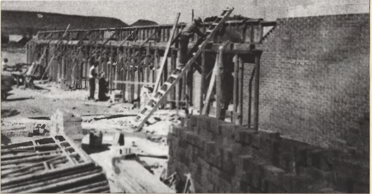
Above: Work on the new College Gymnasium, located on 700 East in St. George, was completed in 1957, but it remained the only building on the new campus until 1961, when the Fine Arts Building was completed.
