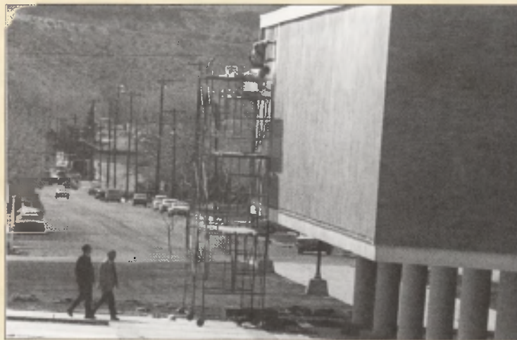
Above: Workers painstakingly place mosaic tiles on the Fine Arts Building facade. The building was completed and ready for classes in 1961, but the mural wasn't added until 1975.
