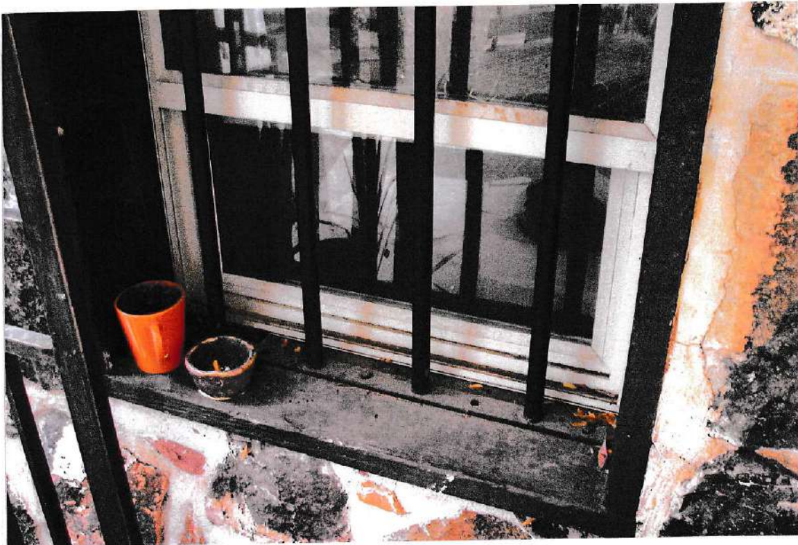
Photograph of the window noted in the above photograph. This photograph shows the iron bars attached to a flat iron plate which has been bolted to the wooden window frame. This would not have been how a jail window would have been built. The bars would have been cemented into the rock structure.
