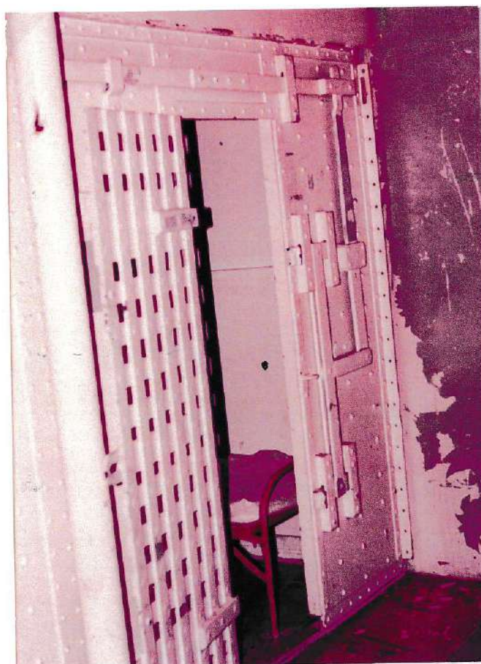
This is a closer view of one of the old cells as it appeared in 1981. Note the Pauly Jail Lever Lock System which secured the cells. Everything was locked together using hot rivets.
