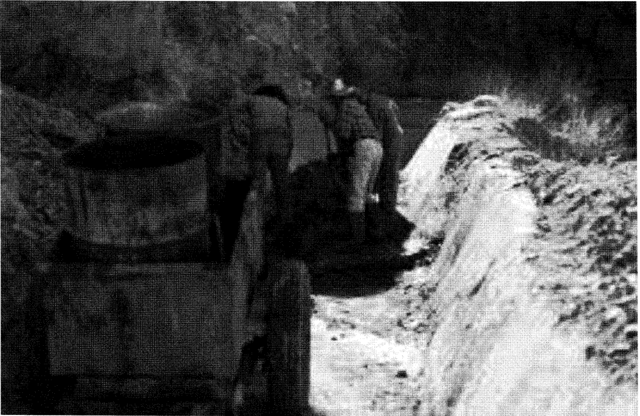
Repairing a break in the Canal just west of the Chinatown Flume
